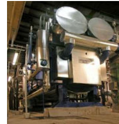
Thisted District Heating 10.5 MW
