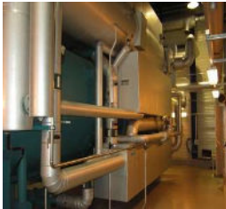
Copenhagen District Heating, Denmark 27.5 MW
